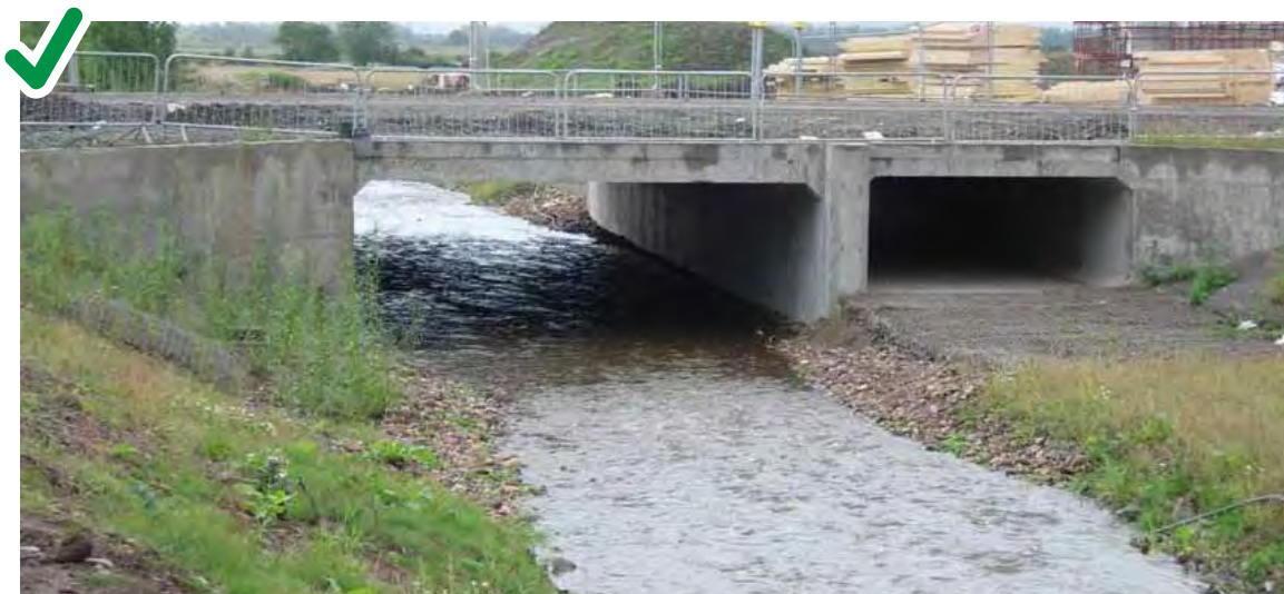
Figure 38: Good practice, culvert maintaining natural channel width, bed level and slope ensuring adequate water depth and water velocity for fish passage.
