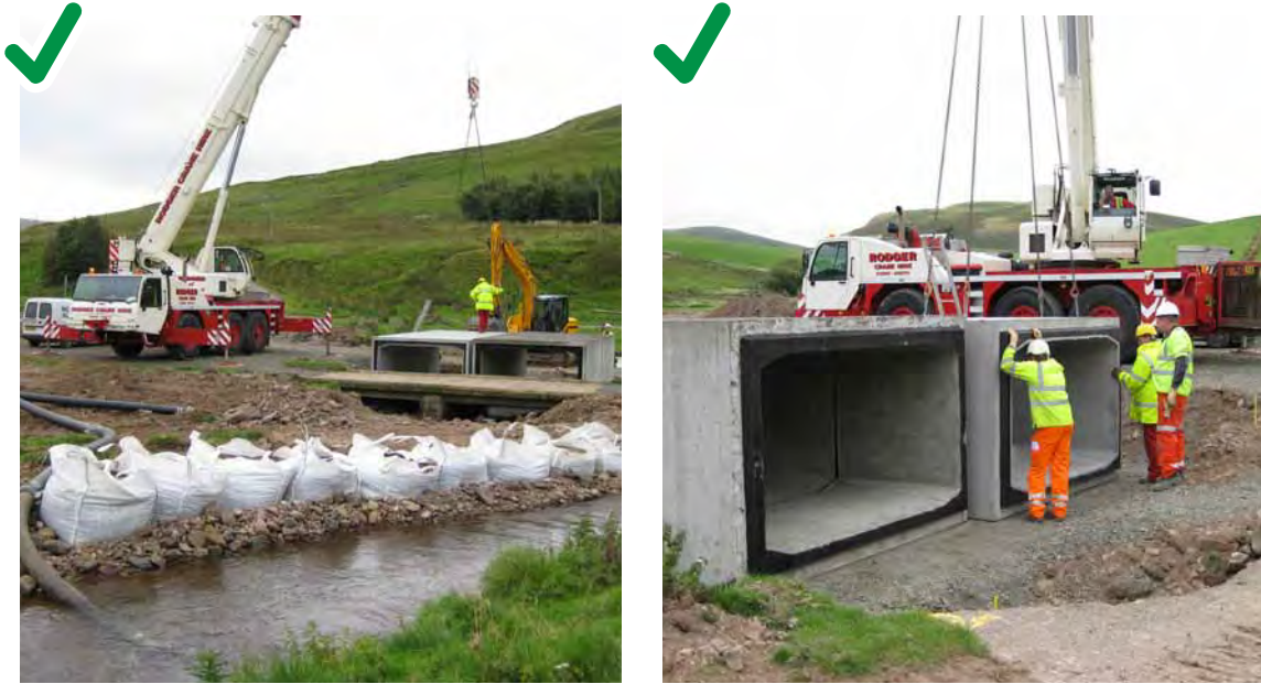
Figure 56: Good practice, works area has been isolated and kept dry by a temporary diversion (left) to allow installation of a culvert (right) that requires working in the river bed.
