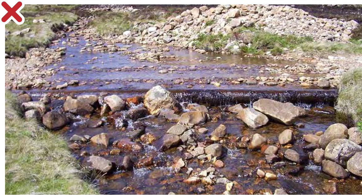
Figure 7: Poor practice. This ford has widened the river, leading to flows that are too shallow for fish to swim through. Photograph courtesy of the River Dee Trust.
