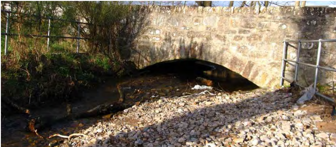
Figure 10: Increased sediment deposition at a bridge can increase flood risk
